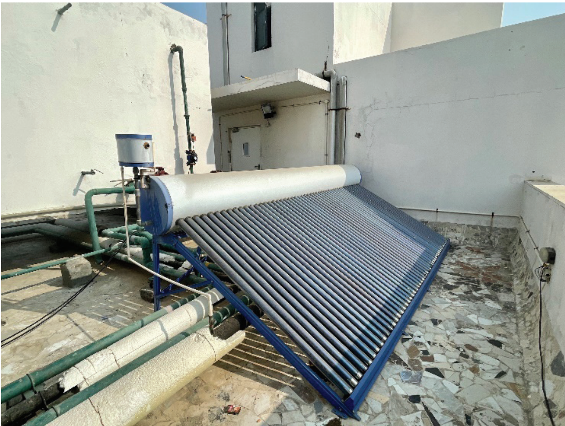
Solar Water heater
