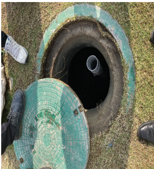
Recharge pit with borewell
