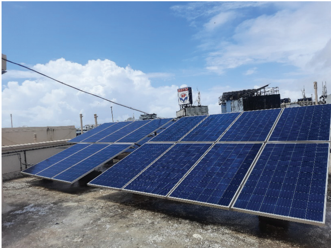
On-site Solar PV
